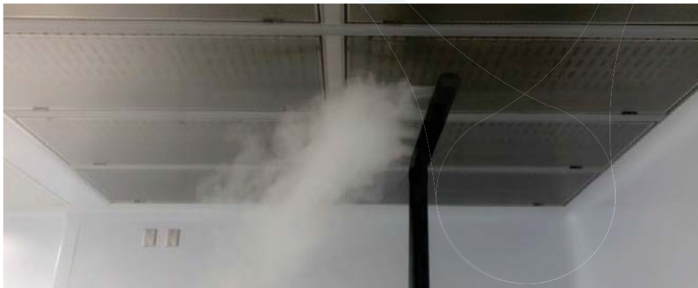
Figure 2: Nitrogen and water “Cleanroom Fogger” Beneath HEPA filters. Note: HVAC is Off
